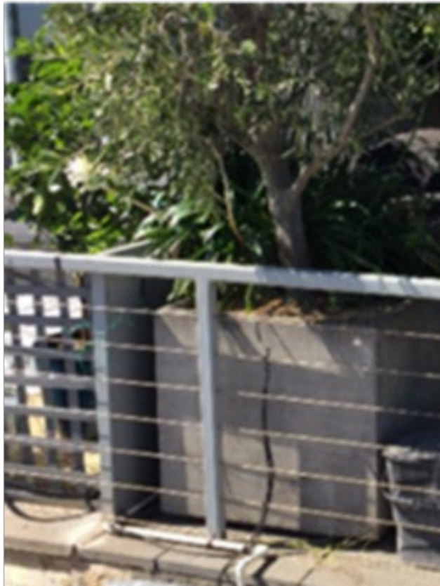
Figure 69: Defect - sagging of handrail (heavy loading)
