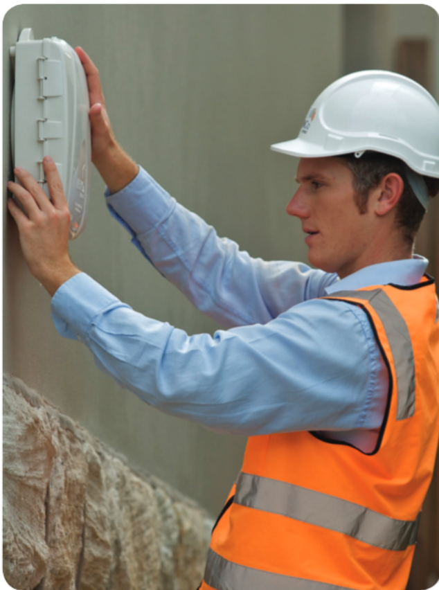
NBN Co or an NBN Co subcontractor will install fibre infrastructure to each premises in a new estate.
